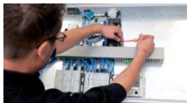
Testing of drives
