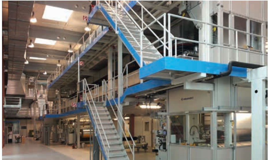
A look at KROENERT's laminating line which was installed at Constantia Teich
